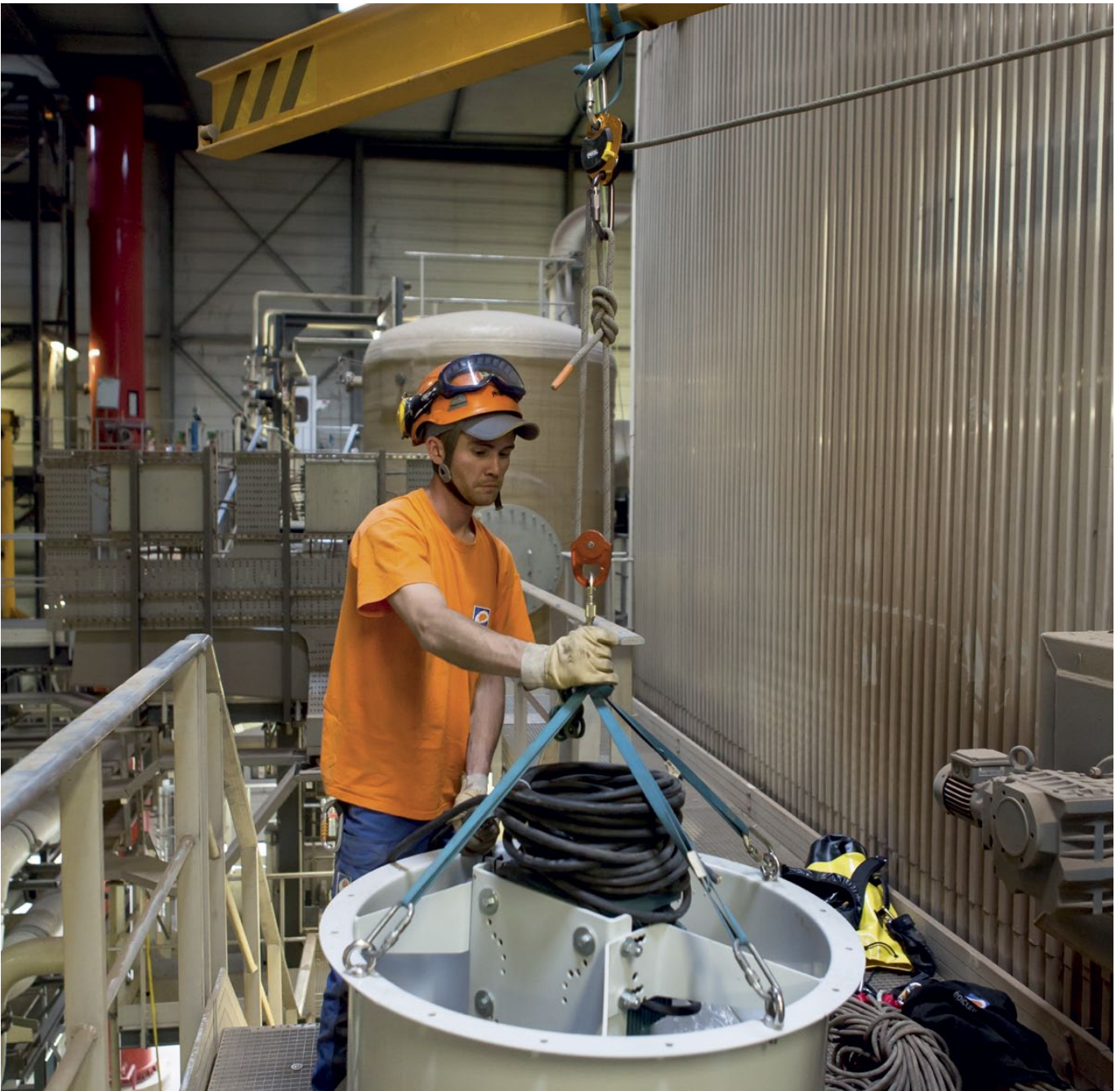
EPICURE, Usine traitement des eaux, Pierre Benite, Rhone, France © Lafouche
