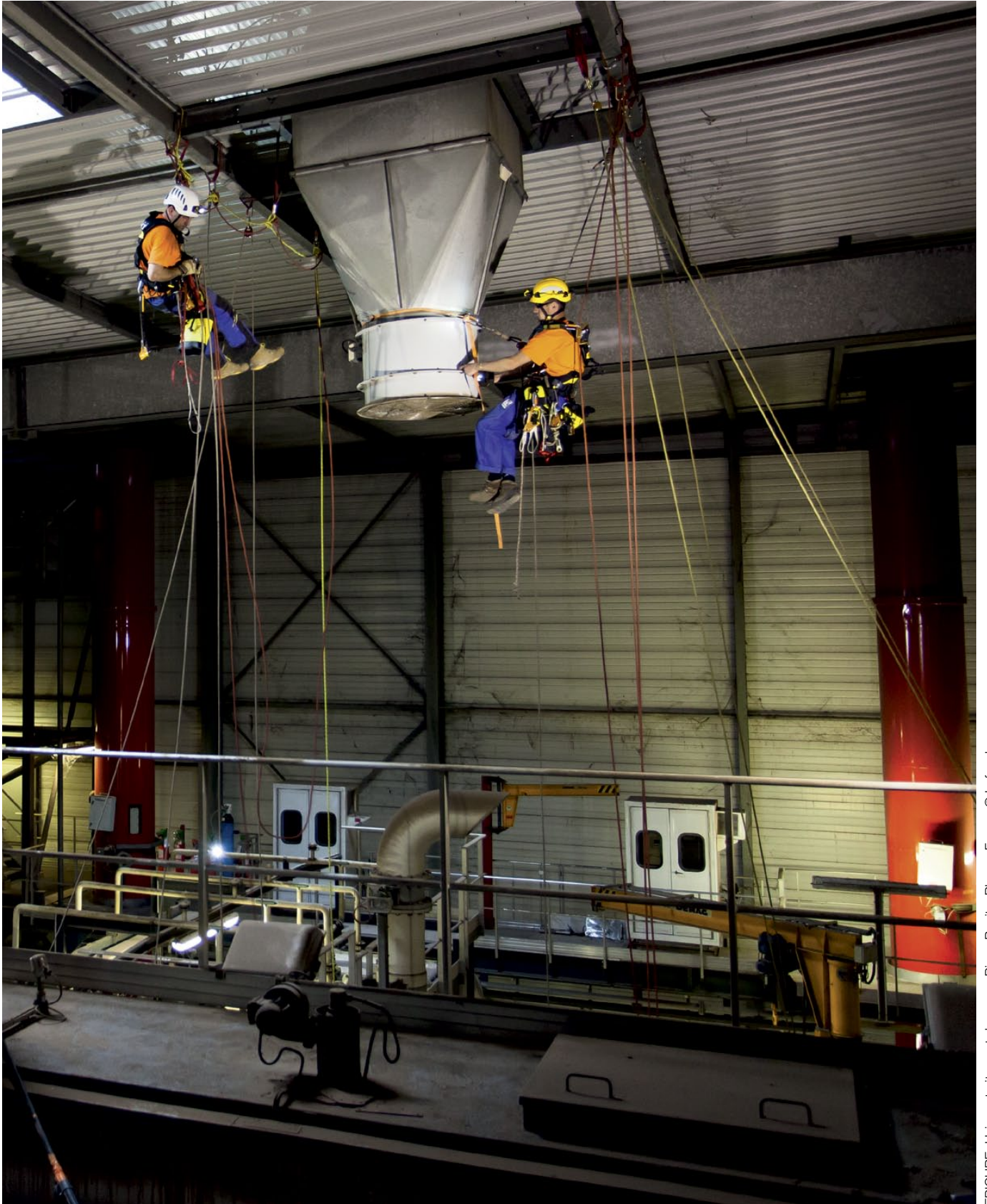
EPICURE, Usine retraitement des eaux, Pierre Benite, Rhone, France © Lafouche
